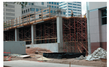
The RRF progresses quickly, with the foundation poured and first floor columns up.
