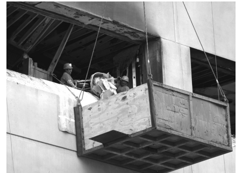
Workers clean up debris caused by Saturday morning's fire at the RRF.
